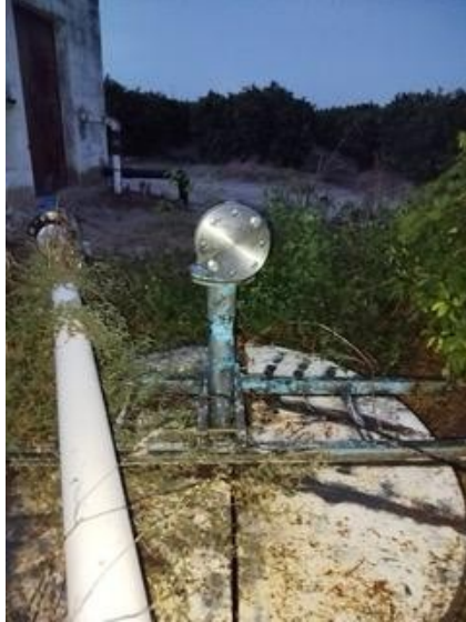
Sealing of a borehole due to lack of legal documentation for it.
